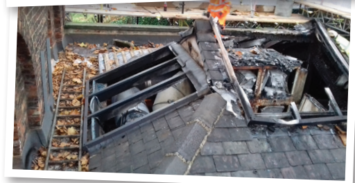
Photos showing the extensive damage caused by the fire.
